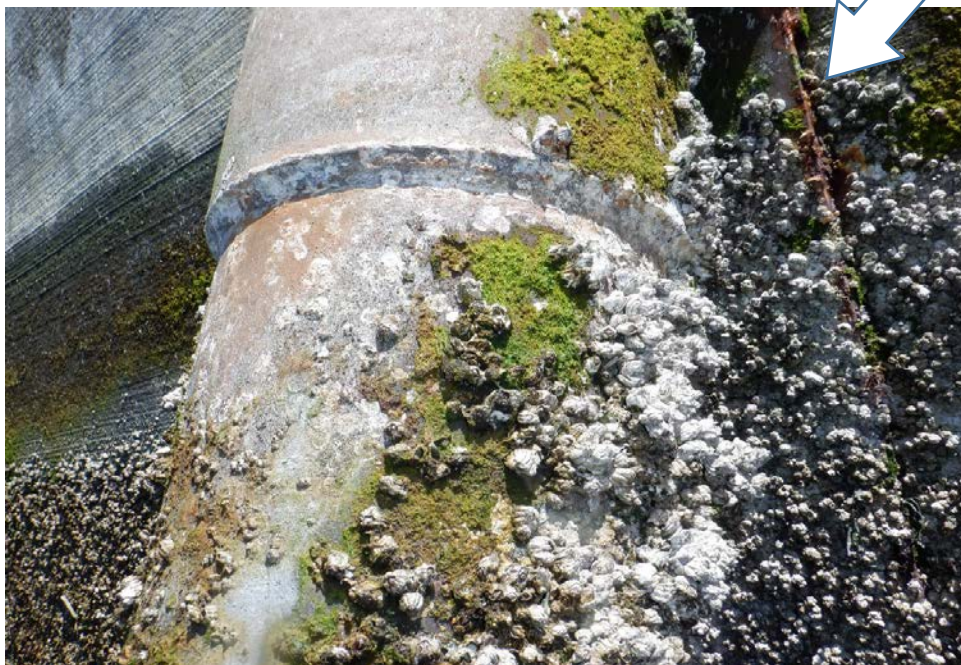
PHOTO No. 14: East Breakwater, Sleeve / Socket Weld - Level II cleaning of the Pipe Sleeve to Pipe Pile socket connection found the welds to be in overall good condition. Also note the corrosion of the H-pile flange (refer to arrow) and the overall good condition of the concrete panel on the left.
