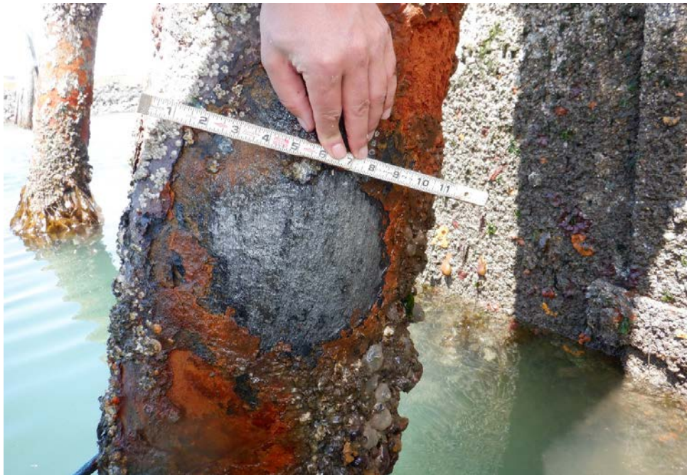
PHOTO No. 21: East Breakwater, Pipe Pile No. 2 Br - Note the bright orange, active corrosion and heavy scale visible on the pile in the lower intertidal zone. Level II cleaning and detailed inspection noted that the base metal is rough with areas of localized pitting.
