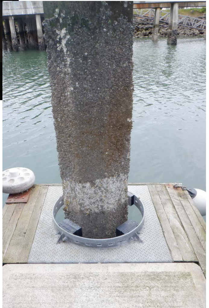
PHOTO No. 6: Float Anchor Pile No. 48, Looking West - Note the area of Level II cleaning visible in the intertidal zone just above the deck. Level II cleaning and detailed inspection was performed on a sampling of the concrete float anchor piles throughout the marina. Also note the typical good condition of the pile hoop and the HDPE rub strips.
