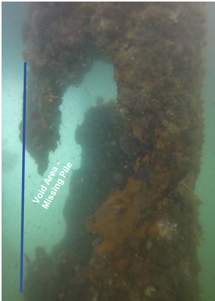
PHOTO No. 22: North Breakwater, Pipe Pile No. 2 Br - Inspection found extensive corrosion, perforation and loss of section on this batter pile. Note the blue line indicating the location of the original pipe pile wall which is now missing. Inspection found nine of the eleven batter piles in the North Breakwater and ten of the 79 batter piles in the East Breakwater to have sustained corrosion to the point of perforation.
