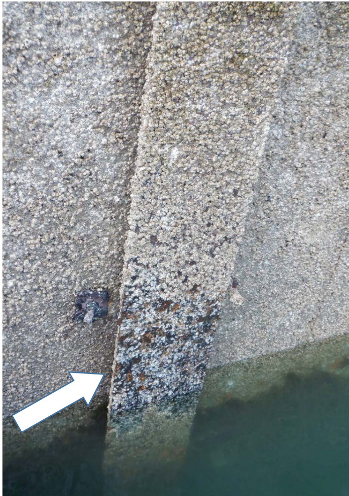
PHOTO No. 17: North Breakwater, Exterior Face, Pile No. 2 - Note the Level II cleaned area on the steel H-Pile at the water surface showing localized failure of the galvanized coating. Also note the gap between the concrete panels and the flanges of the H-Pile (refer to arrow). The concrete panels are flush with the H-Pile flanges on the inside face of the breakwater.
