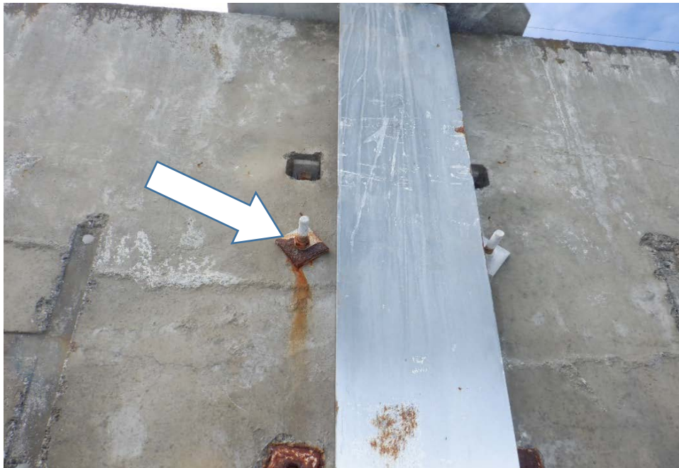
PHOTO No. 12: Breakwater, Exterior Face, Typical Condition - Note the corrosion evident on the connection hardware which secures the concrete panel (refer to arrow). Also note the overall good condition of the protective coating on the H-Pile in the splash zone.
