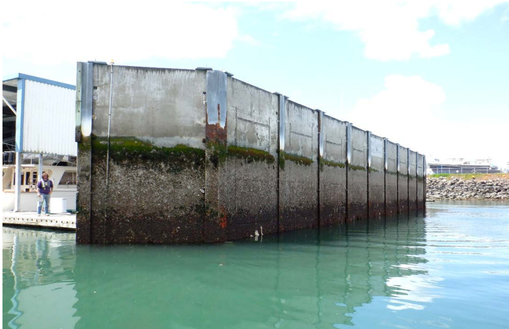
PHOTO No. 9: North Breakwater, Looking West - This is one of two smaller breakwaters that protect the entrance to the marina. Both are constructed with 11 sets of vertical steel H-piles with a steel pipe pile batter, with inset concrete panels extending from the top of the breakwater to the mudline.
