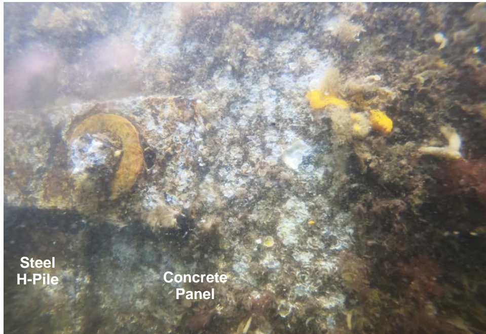
PHOTO No. 18: North Breakwater, Interior Face, Concrete Panel Connection Plate - Note the Level II cleaning of the concrete panel and the steel plate connection bracket. The concrete was found to be in overall good condition, while moderate surface corrosion is visible on the steel plate and hardware.
