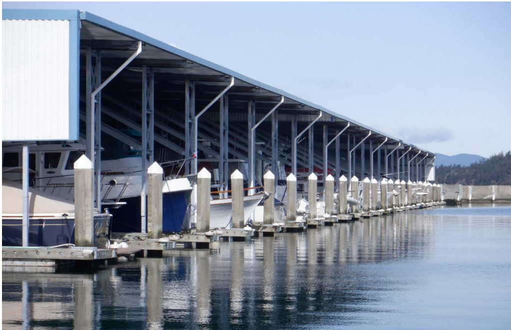
PHOTO No. 3: Marina Moorages, West Edge, Looking North - Note the good condition of the concrete piles and floats in this area. Also note the north end of the East Breakwater visible in the background.
