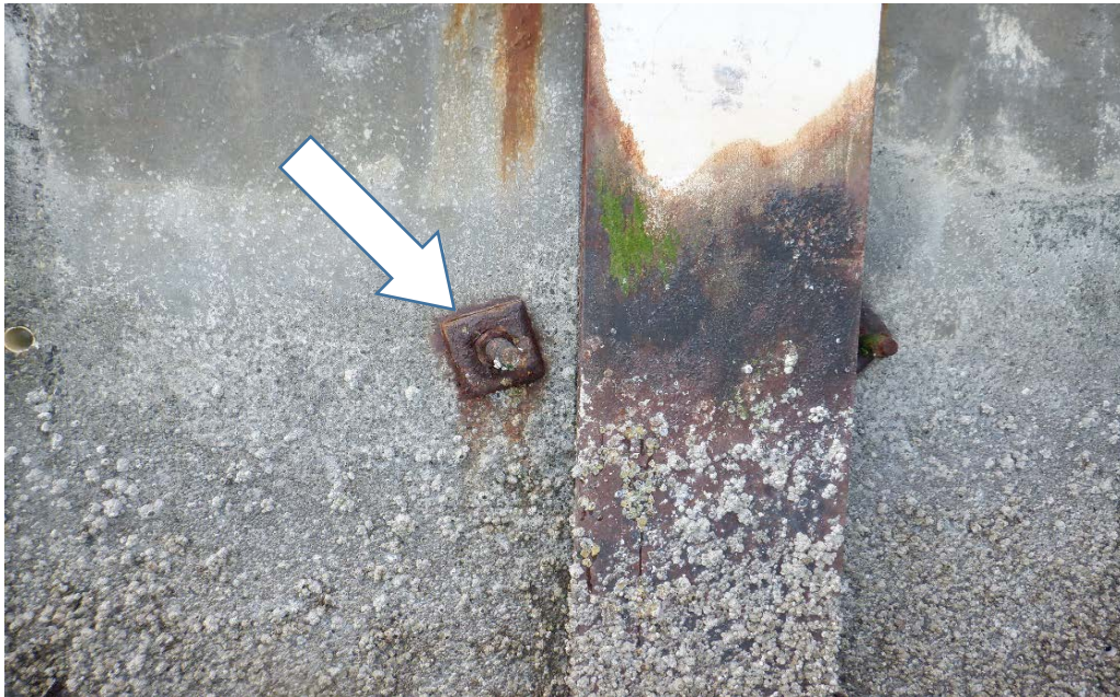
PHOTO No. 15: Breakwater, Exterior Face, Typical Condition - Note the moderate to heavy corrosion and scale of the attachment hardware which serves to secure the concrete panels to the H-Piles (refer to arrow). Also note the failed coating and corrosion of the pile from the high tide down and the overall good condition of the coating above. This was found to be typical of the piles throughout both breakwaters.
