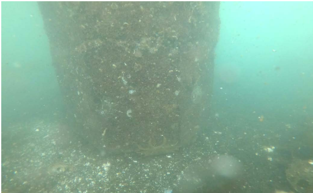
PHOTO No. 7: Float Anchor Pile No. 10 - Note the overall good condition of the concrete pile with well defined corners and no evidence of any cracking, spalling or rust bleeding. Also note the silty-sand and gravel composition of the mudline. Both of these conditions were found to be typical of the float anchor piles throughout the marina.
