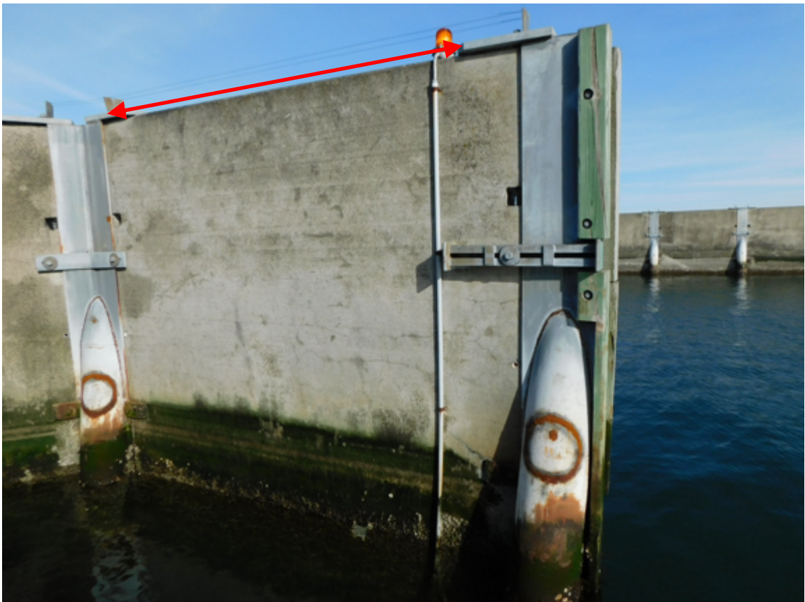
Electrical potential measurement between adjacent supports to determine electrical continuity
