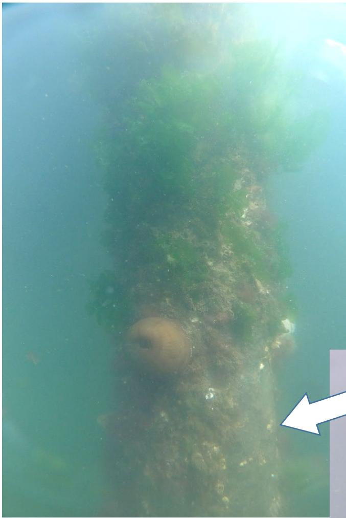
PHOTO No. 5: Batter Pile No. 38 - Note the generally good condition of the pile in areas which are not covered by marine growth (refer to arrow). Also note the lack of active orange surface corrosion on the pile.
