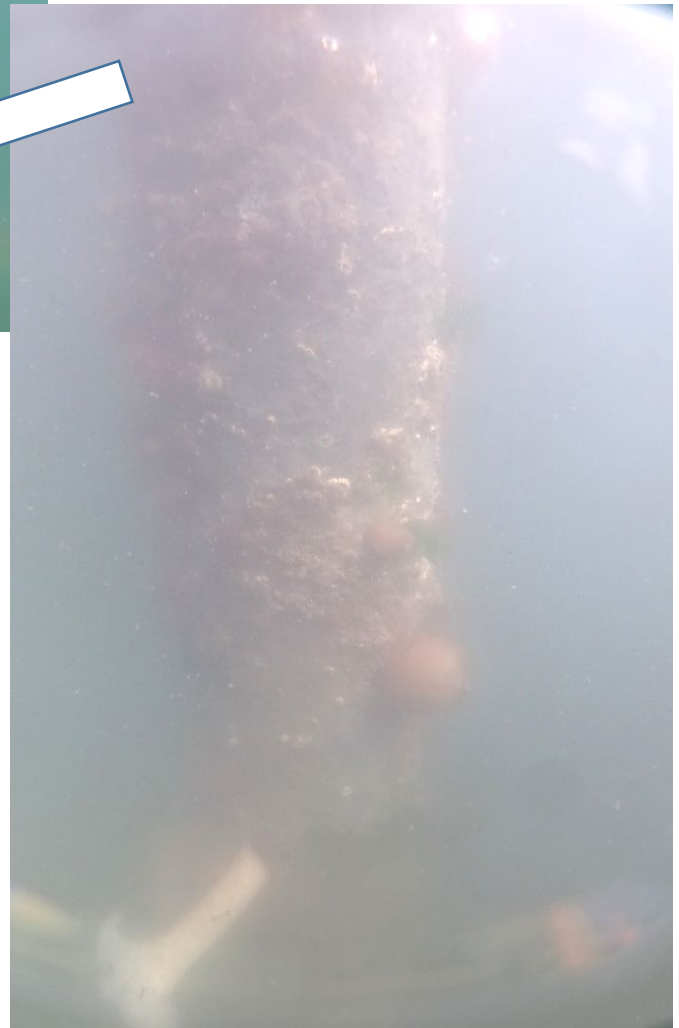
PHOTO No. 6: Batter Pile No. 38 - Visual investigation of the piles along with the data obtained from the Corrosion Potential survey, found the batter piles to be protected from on-going corrosion. These conditions were typical of the inspected piles with no evidence of active surface corrosion noted.
