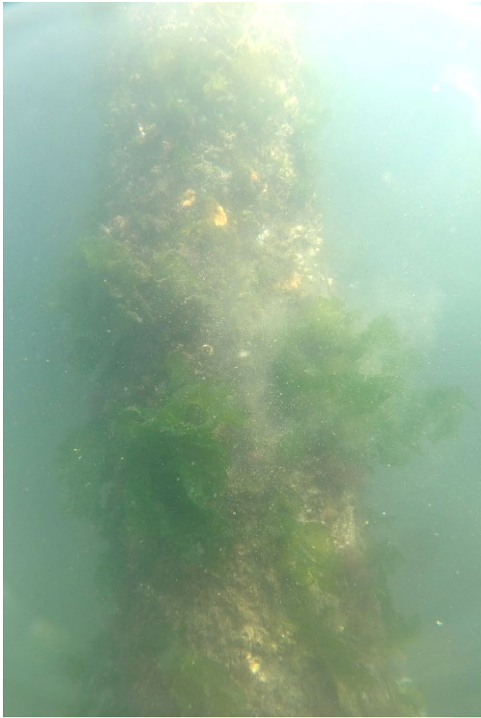
PHOTO No. 3: Batter Pile No. 27 - Note the moderate marine growth on the pile in the lower intertidal zone. Also note the lack of bright orange surface corrosion which was evident on the pile during the previous 2021 inspection.
