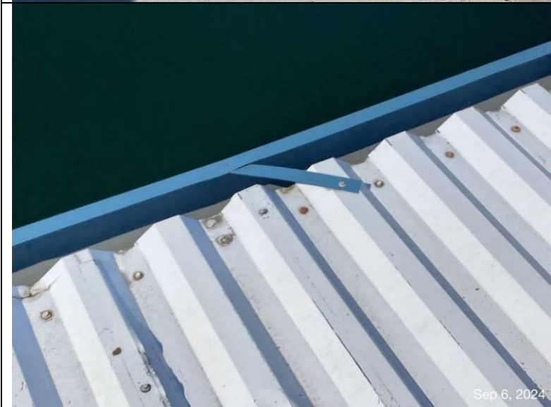
Photograph 60: View of loose gutter straps with missing fasteners.
