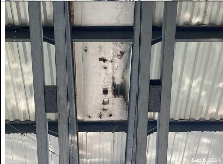
Photograph 47: View of damaged condensation blanket.
