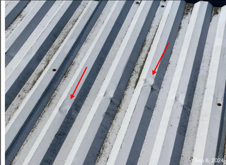
Photograph 56: View of damaged roof panels with slight corrosion.
