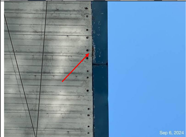
Photograph 54: View of roof panel eave edge corroded at the fastener penetrations, as well as corroded gutter edges.
