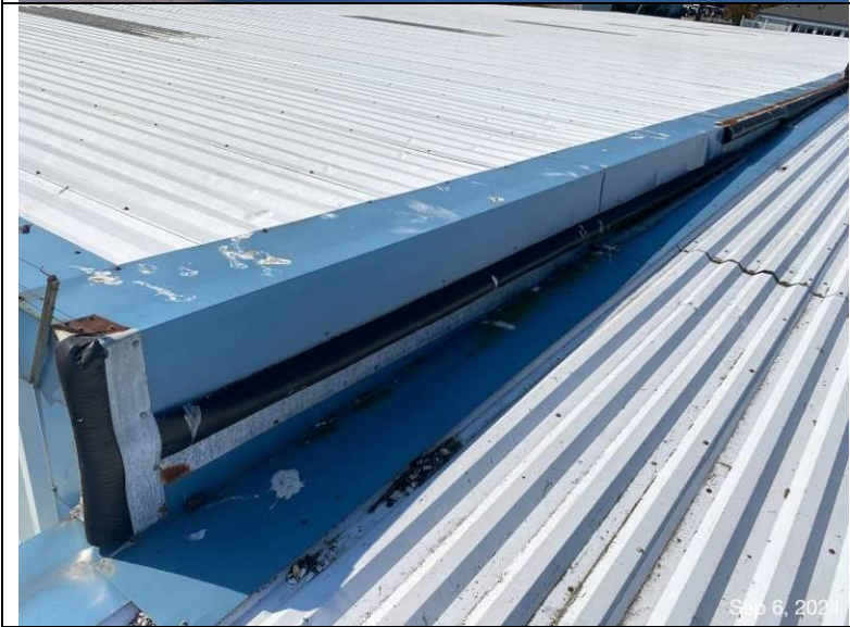
Photograph 33: View of the expansion joint at the northeast corner of the south roof.
