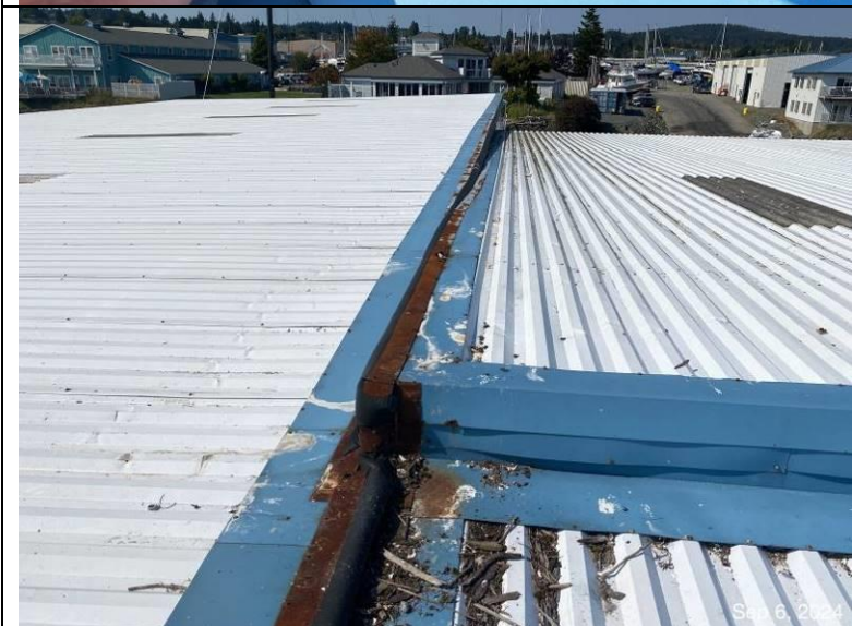
Photograph 36: View of the expansion joint between the south and north roof areas.
