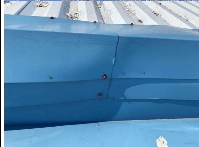
Photograph 30: View of the rake flashing secured directly through the laps causing the metal to buckle.
