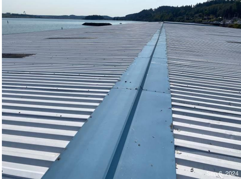
Photograph 24: View of the ridge flashing mechanically fastened to the top flutes of the roof panels.
