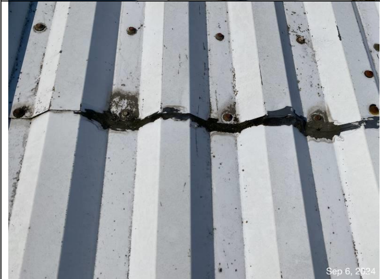
Photograph 53: View of end lap of the field roof panel lifted and sealed with sealant.
