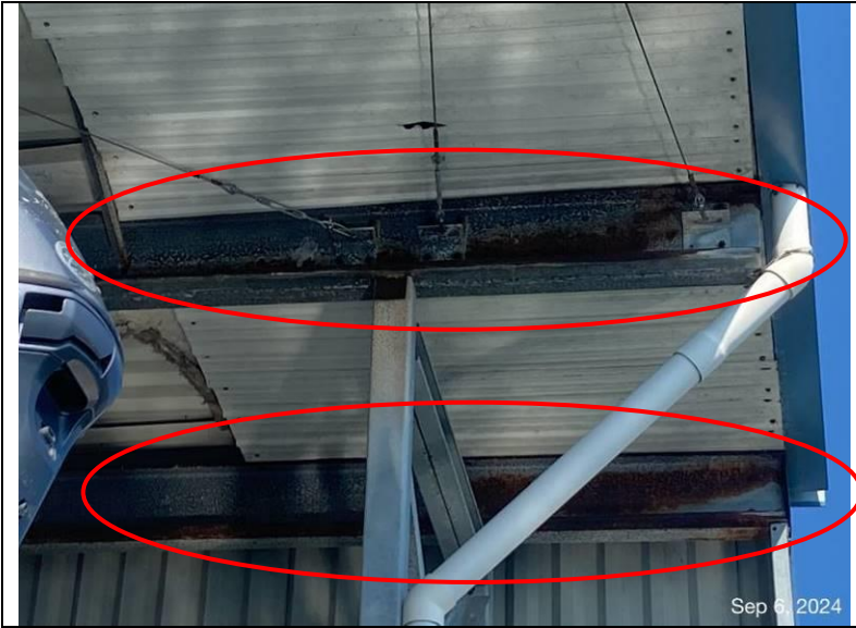
Photograph 61: View of surface corroded steel beams.
