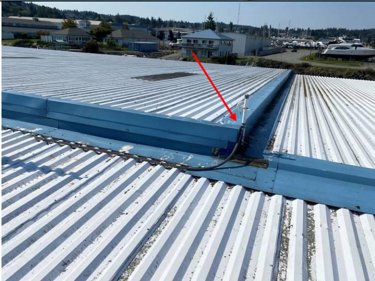
Photograph 42: View of an antenna penetration at the roof plane change, secured through the roof-to-wall transition flashing.
