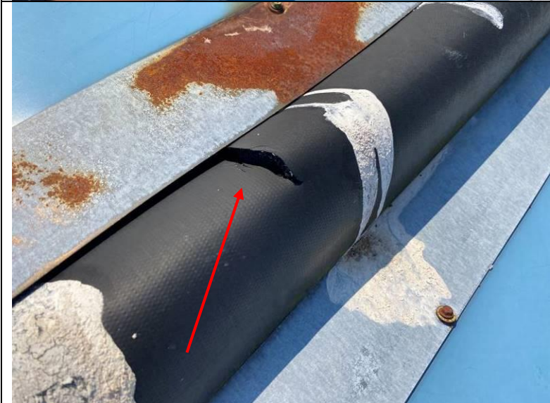
Photograph 38: View of damage in the expansion joint membrane.
