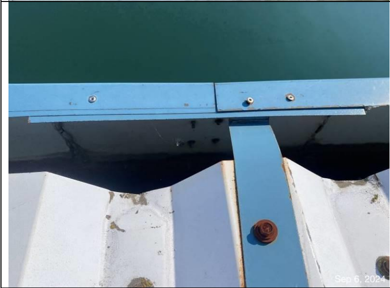
Photograph 18: View of gutter laps with flat plate on the inside of the gutter, embedded in sealant and secured with rivets.
