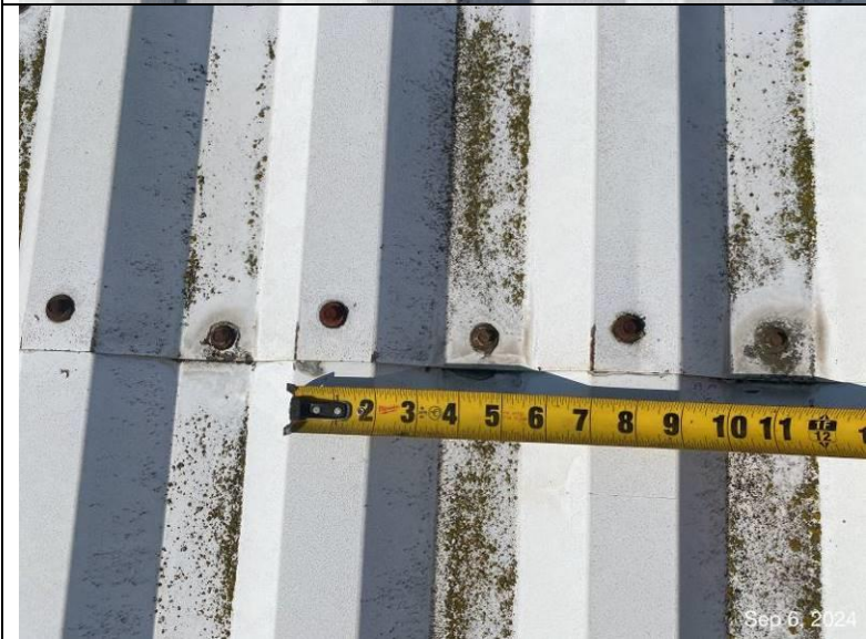
Photograph 12: Fastener spacing at the overlaps of the roof panels measuring at approximately 4-inches on-center.
