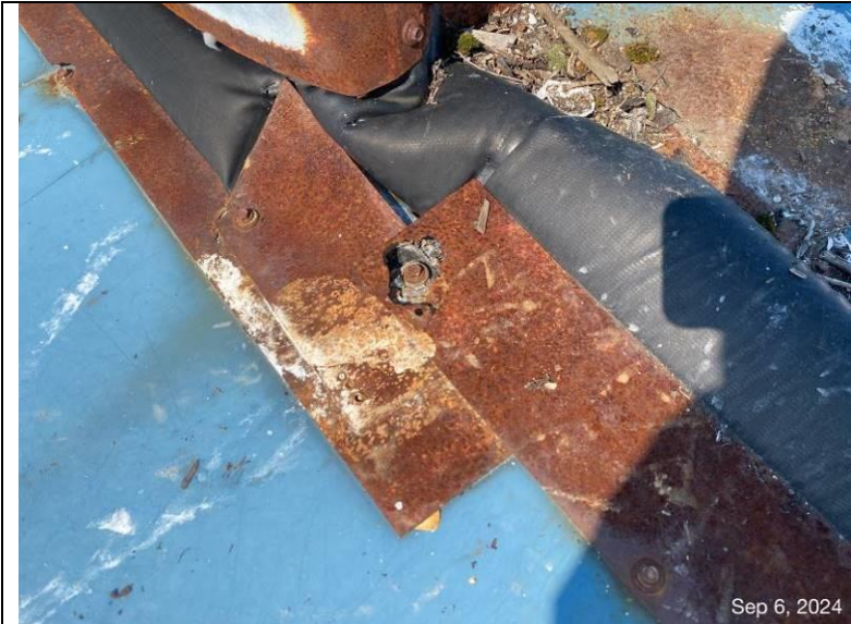
Photograph 40: View of corroded expansion joint flanges.
