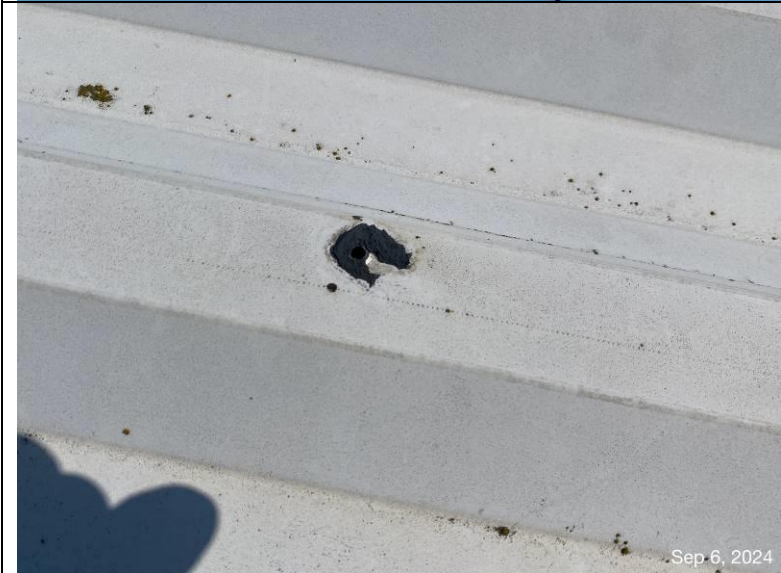
Photograph 59: View of missing fastener in the field of the roof panel.
