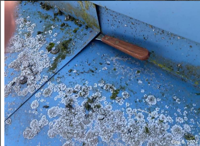
Photograph 29: View of sealant knife fully inserted into the lap of the roof-to-wall flashing.
