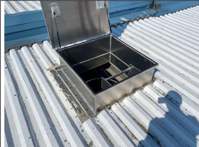
Photograph 4: View of the access to the roof through a hatch, centrally located on the east slope.
