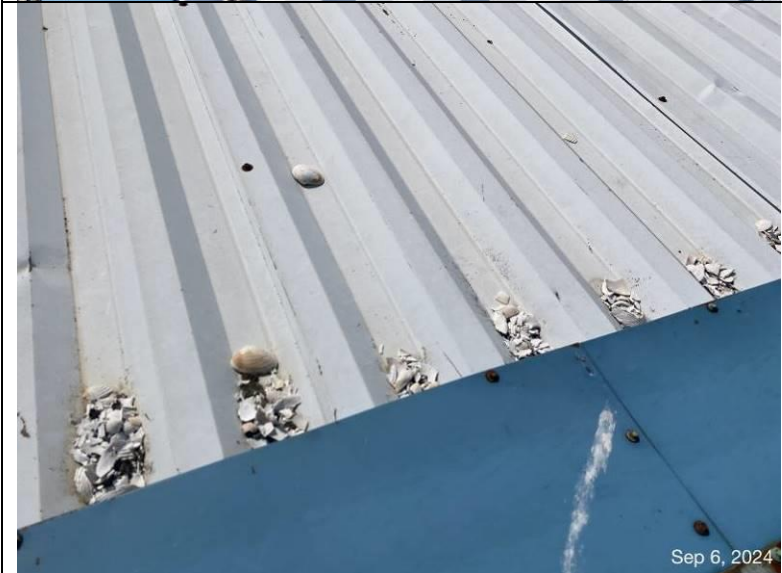
Photograph 65: View of seashells on the roof.
