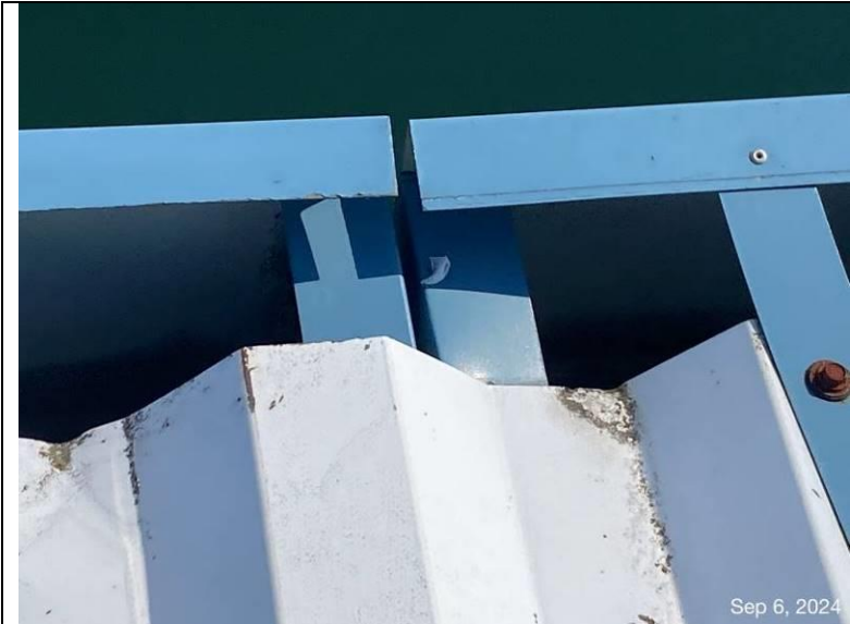
Photograph 19: View of the gutter expansion joint without a cover.
