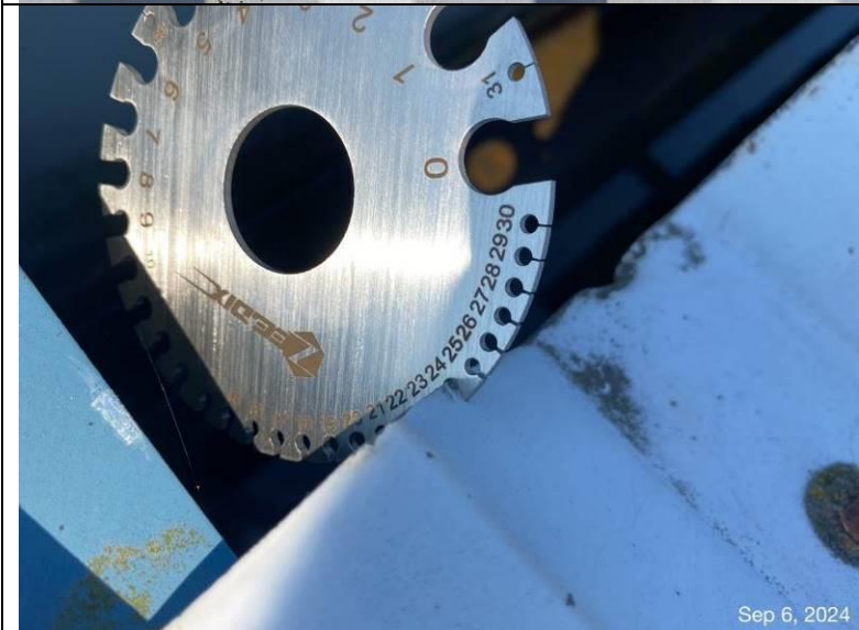
Photograph 14: Metal roof panels with a metal gauge inserted at the end of the panel measuring at 24-gauge.
