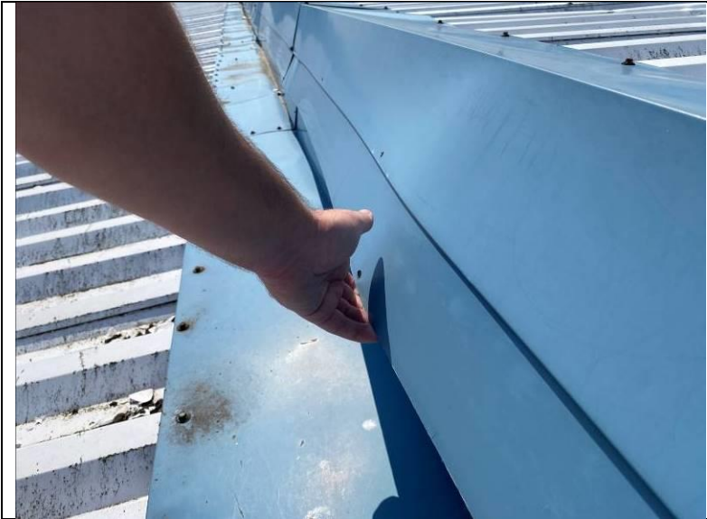
Photograph 31: View of missing fasteners at the rake to roof-to-wall overlap.
