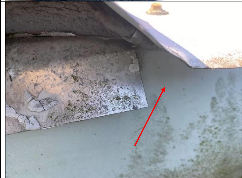
Photograph 17: View of the gutter flange under the metal roof panels. Note the flashing at the eave of the roof extending into the gutter missing at some locations.
