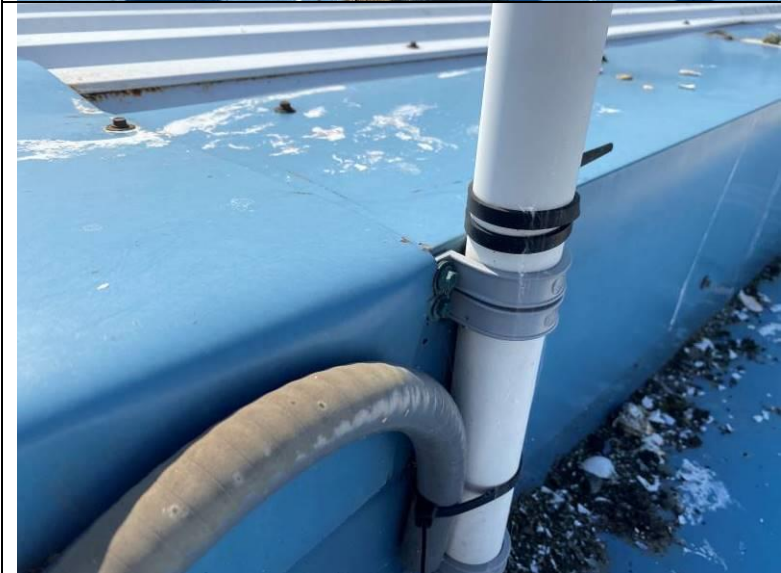
Photograph 44: View of an antenna penetration secured through the roof-to-wall transition flashing with neoprene gasketed fasteners.
