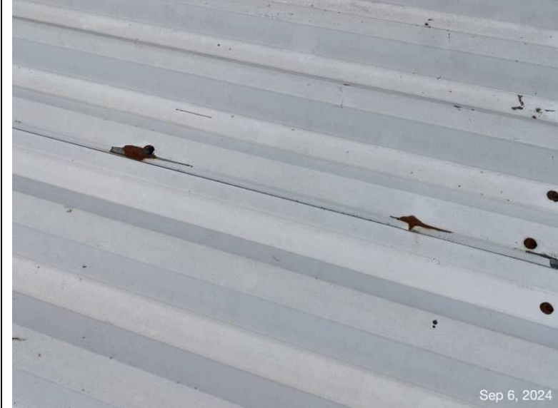
Photograph 57: View of damaged roof panels with slight corrosion.
