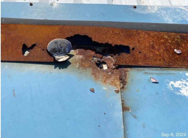
Photograph 41: Alternative view of corroded expansion joint flanges.
