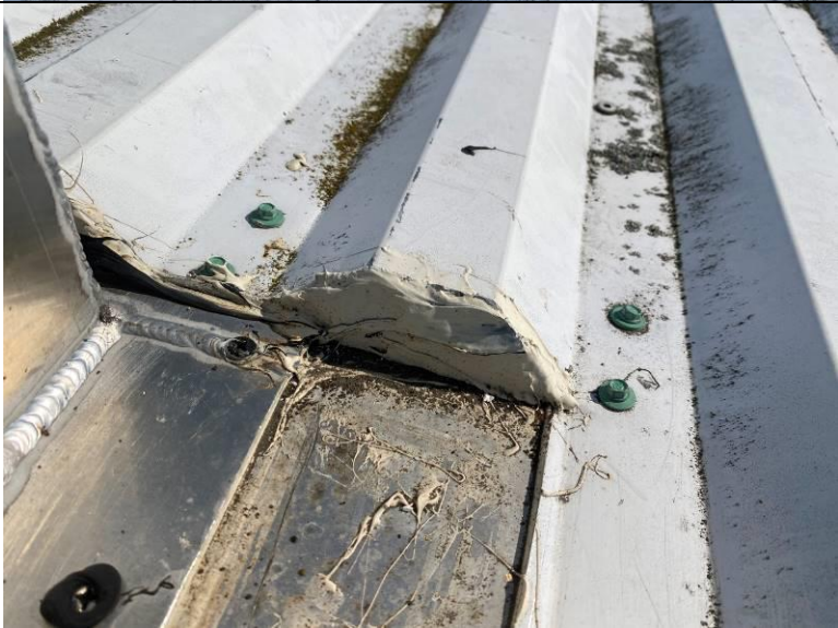
Photograph 6: View of the open edge of the roof panels below the hatch infilled with sealant.
