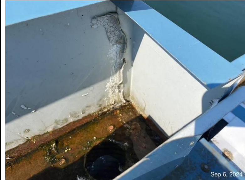
Photograph 20: View of the end of the gutter with the closure plate sealed with sealant.
