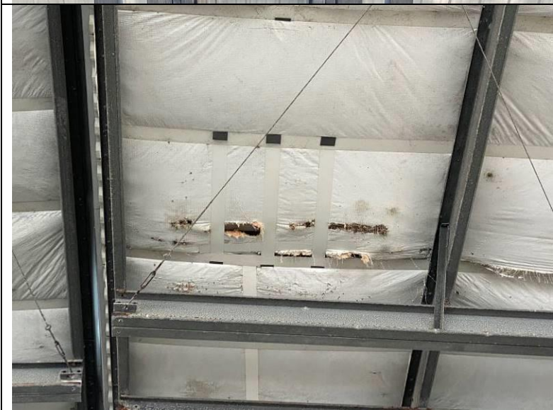
Photograph 48: Alternative view of damaged condensation blanket.
