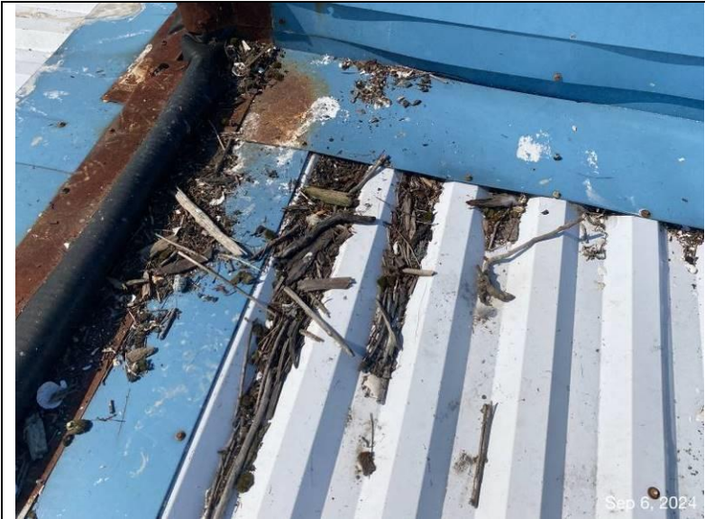
Photograph 64: View of debris pile-up on the roof.
