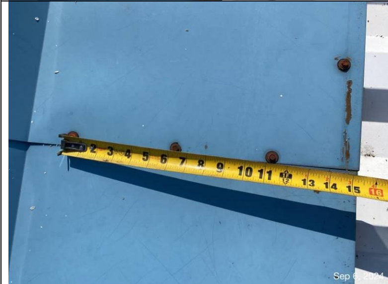
Photograph 26: View of the ridge flashing secured directly through the laps at approximately 6-inches on-center, not allow for expansion/contraction. Note corrosion of fasteners.
