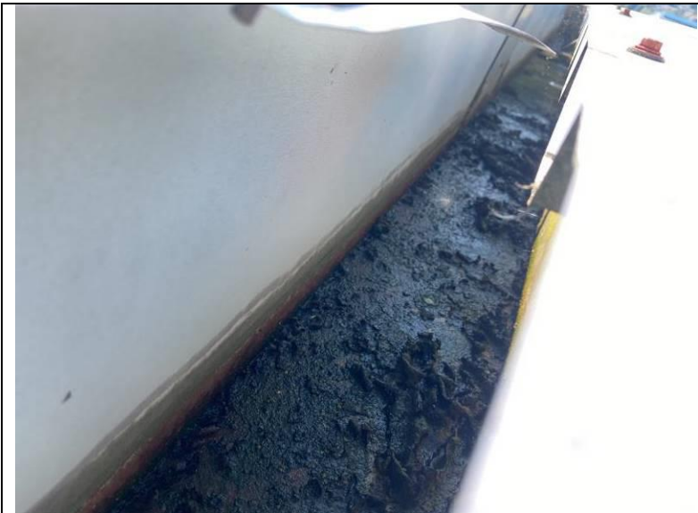
Photograph 16: View of the inside of the gutter, including debris and corrosion along the bottom surface.
