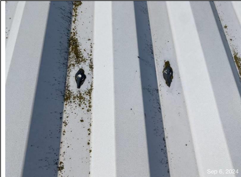
Photograph 49: View of the fasteners in the field of the roof sealed with sealant.
