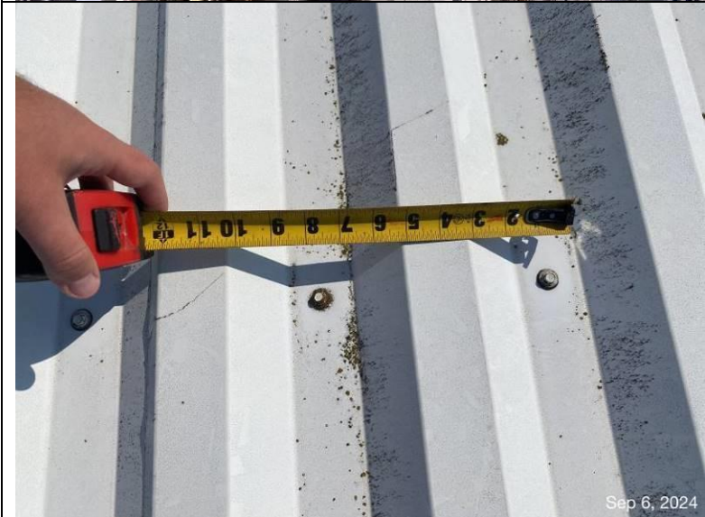
Photograph 11: Fastener spacing in the field of the roof panels measuring at approximately 8-inches on-center.
