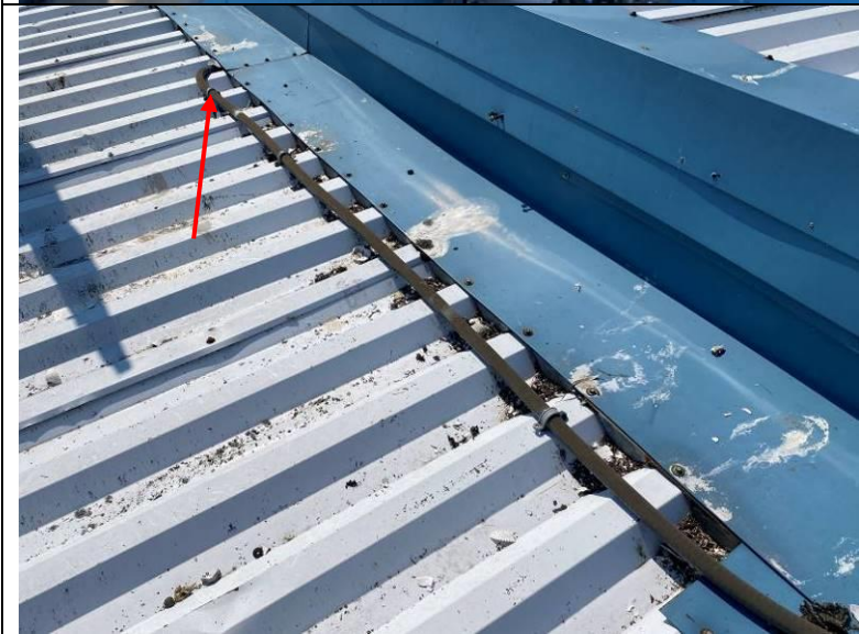
Photograph 45: View of the antenna conduit extending under the roof-to-wall transition.
