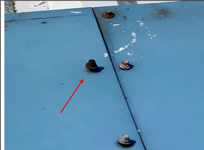
Photograph 58: View of fasteners backing out at the ridge of the roof.
