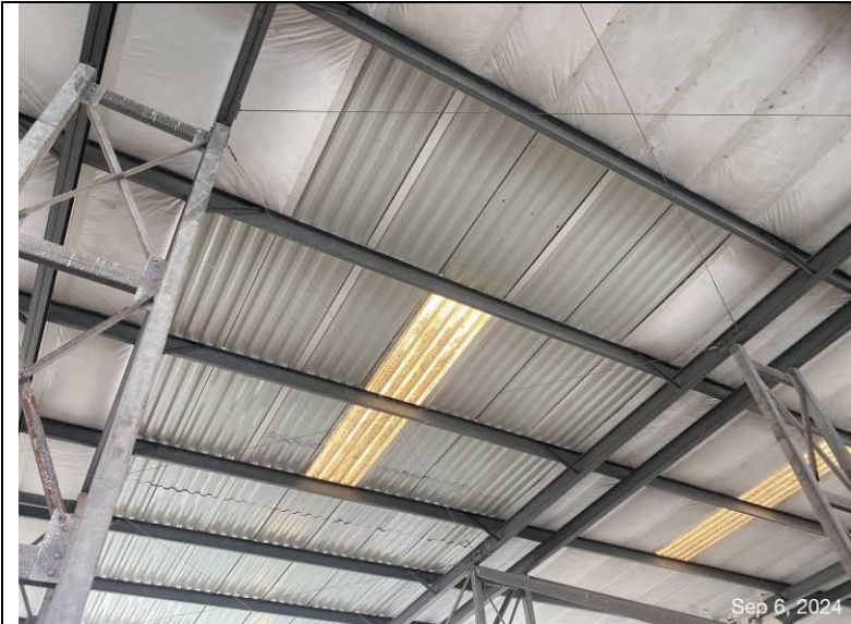
Photograph 46: View of the underside of the roof panels with condensation blanket removed at some locations.
