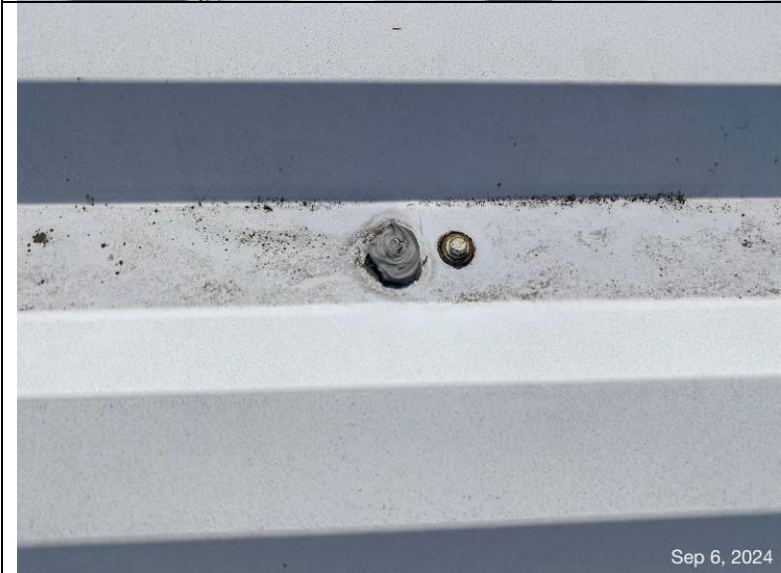
Photograph 50: View of the fasteners in the field of the roof sealed with sealant and a new fastener placed adjacent to the old fastener.
