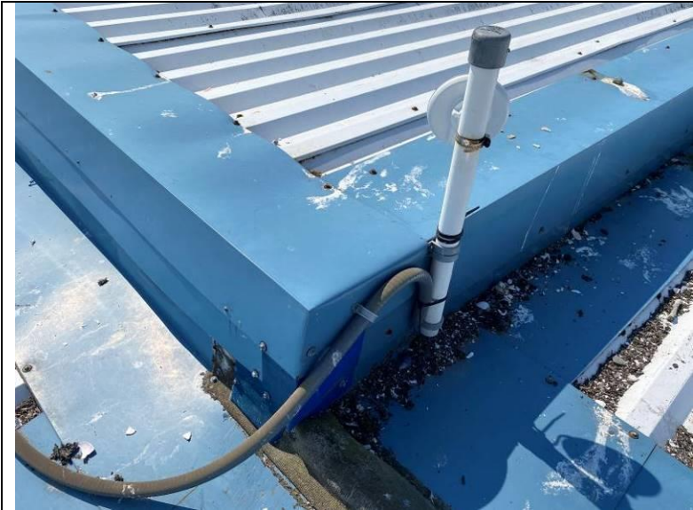
Photograph 43: Close-up view of an antenna penetration.
