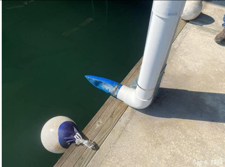
Photograph 23: View of the downspout discharging into the marina.
