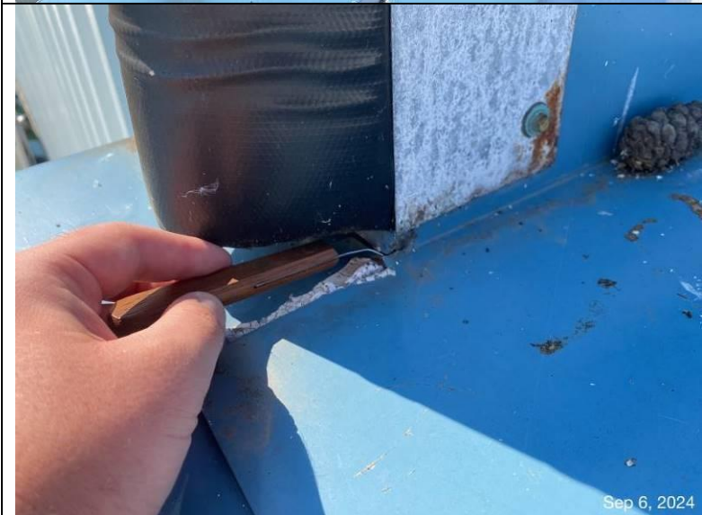
Photograph 35: View of sealant knife inserted into plane transition corner, indicating saddle flashings were not installed.
