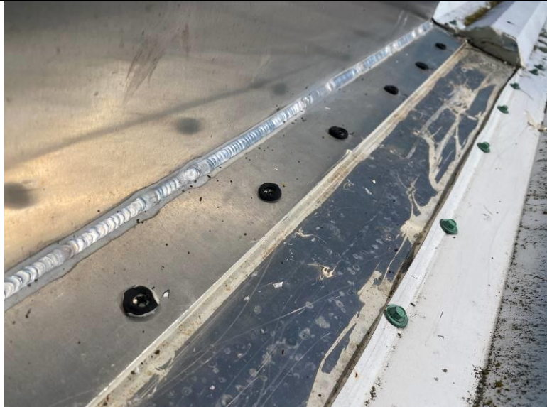
Photograph 7: View of the roof hatch flanges secured through a flat plate with non-gasketed screws embedded in sealant.
