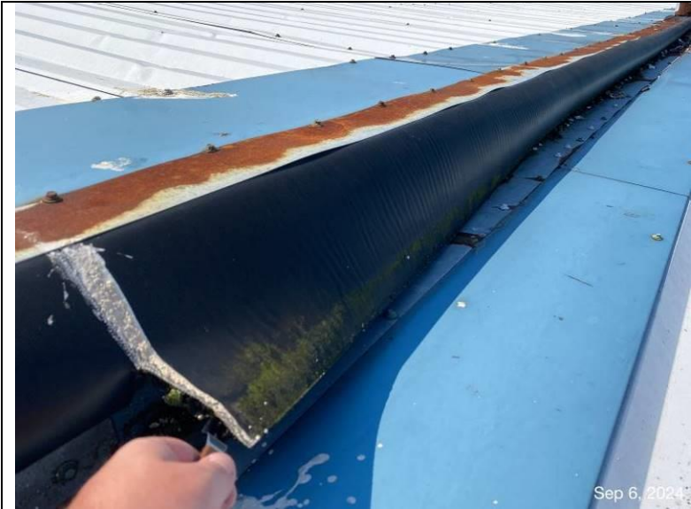
Photograph 37: View of open laps in the expansion joint membrane.
