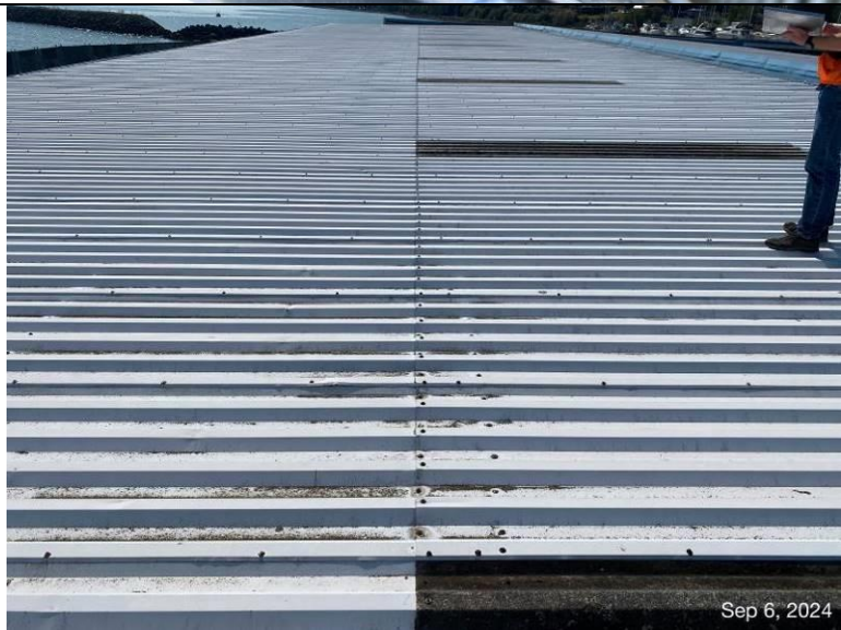
Photograph 9: View of the field of the roof, showing metal and translucent roof panels.
