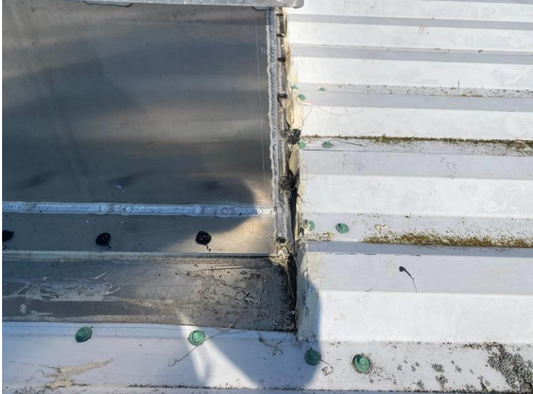
Photograph 5: View of the downslope flange of the hatch extending under the roof panels.
