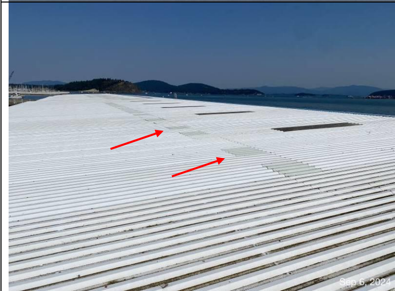
Photograph 51: View of the roof with supplemental roof panels, reportedly installed when several panels stored on the roof blew off during 1996 roof replacement. Note the color difference.
