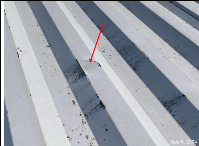
Photograph 55: View of damaged roof panels with slight corrosion.
